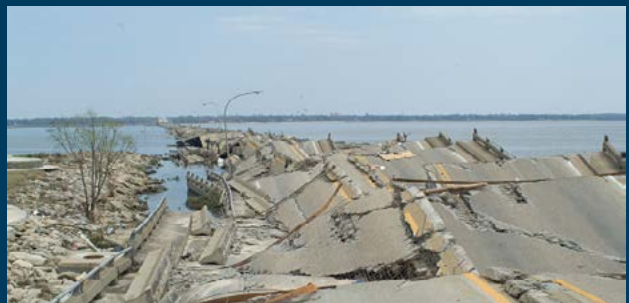
— A portion of Highway 90 in Mississippi destroyed by Hurricane Katrina. Source: Getty Images North America.
